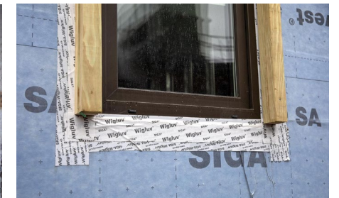
Blue air barrier wrap and sealing tape around high performance uPVC windows
